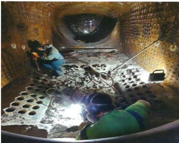
Volunteers remove firebrick from the firebox and the superheaters from the boiler of 2-10-2 #5511
